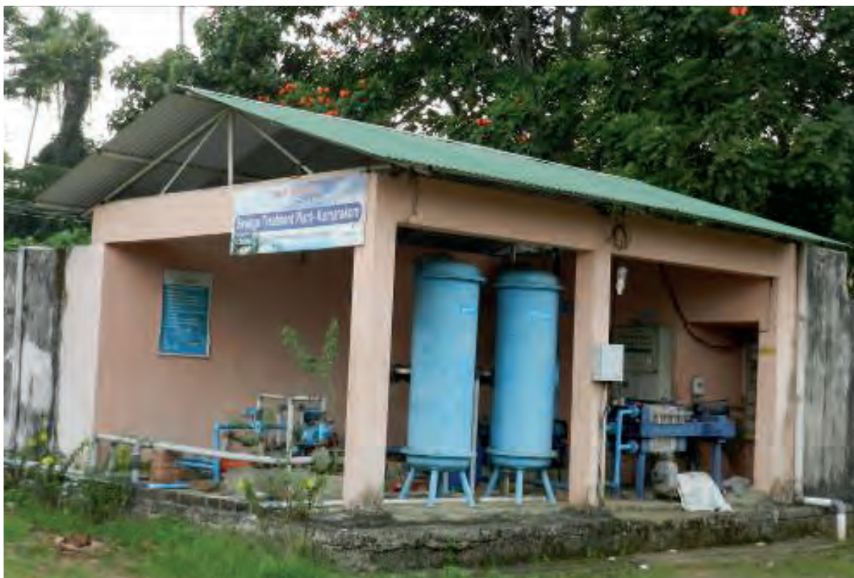
Sewage treatment plant at Kumarakom
